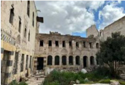
Figure 15. This field photo illustrates damaged building over the cultural site Bayt Ghazale by the Syrian Directorate-General of Antiquities & Museums (DGAM)
