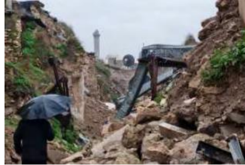
Figure 16. This field photo illustrates damaged building in area between Suq al-Attarin and Suq al-Ebi, Ancient City of Aleppo by the Syrian Directorate-General of Antiquities & Museums (DGAM)
